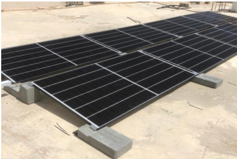
Figure 4a: Solar PV system.
