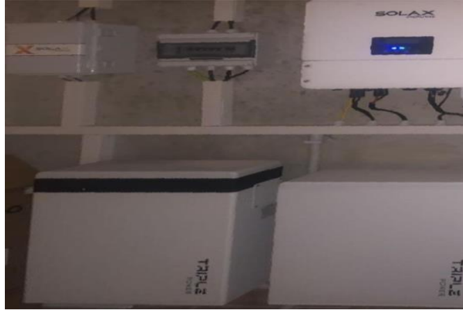
Figure 4b: Solar PV system.
